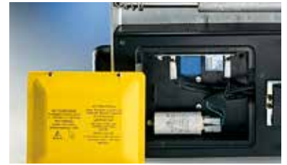
Sealed electrical enclosure
